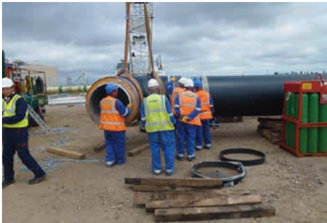
Figure 2. Engineers prepare to fabricate large diameter pipework on the Isle of Grain natural gas installation using QuickPurge.
